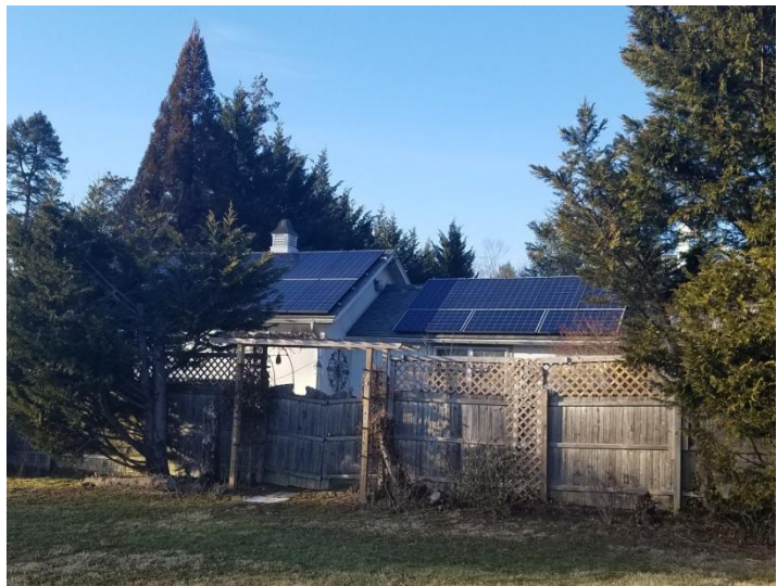
Figure 5-4. Solar PV Panels
